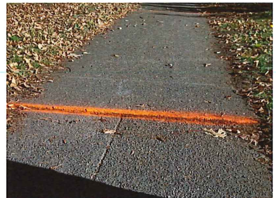
Cracks can be trip hazards.
