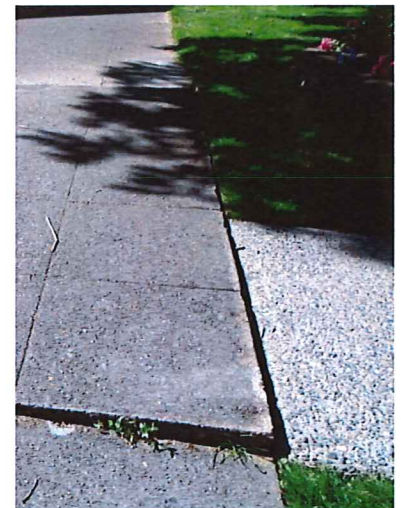
Lifted sidewalks can also pose a hazard.
